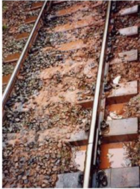
Figure 7: The end result of pumping erosion
