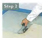
Applying polymer modified cement-based flexible tile adhesive, spreading with an 8mm notched trowel
