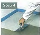
Spreading polymer modified cement-based tile adhesive with an 8mm notched trowel on to Acoustic-si
