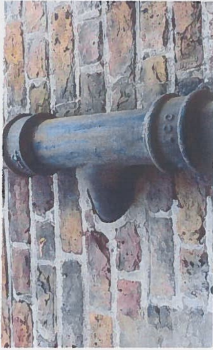
From 2011 showing the original pipework in the same area prior to the Applicant's works
