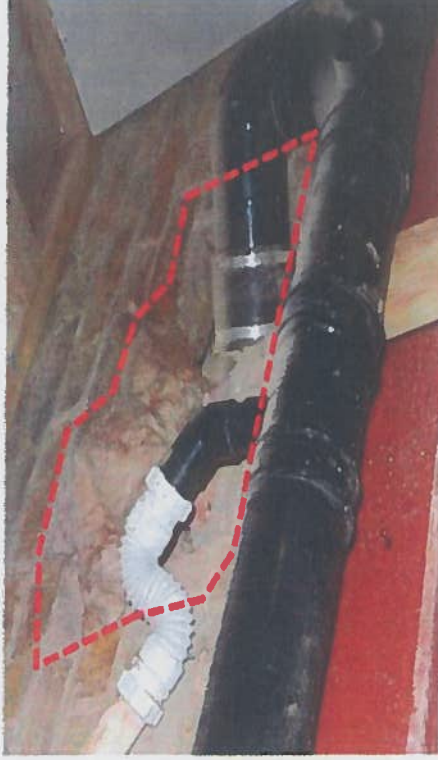
PHOTOGRAPH C From 2014 showing the pipework already damaged by the Applicant's contractor and filled with insulation
